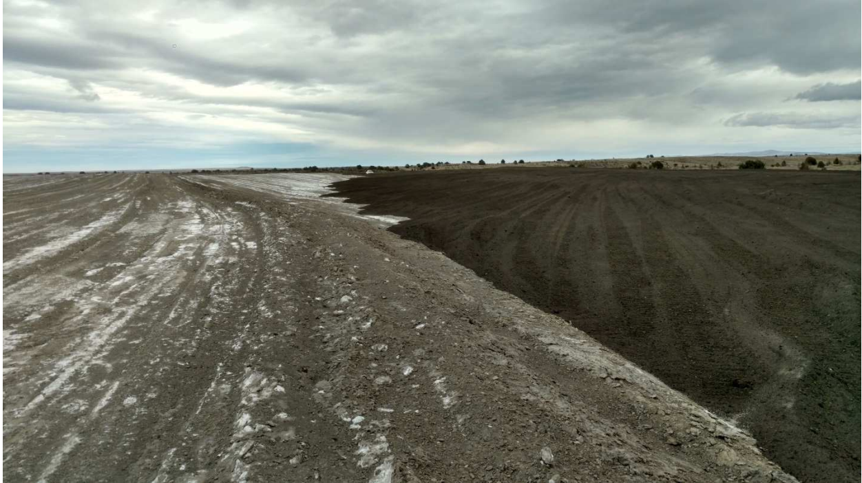
Completed grading of bottom ash to form slopes to be graded and filled with new ash to form uniform pile.
