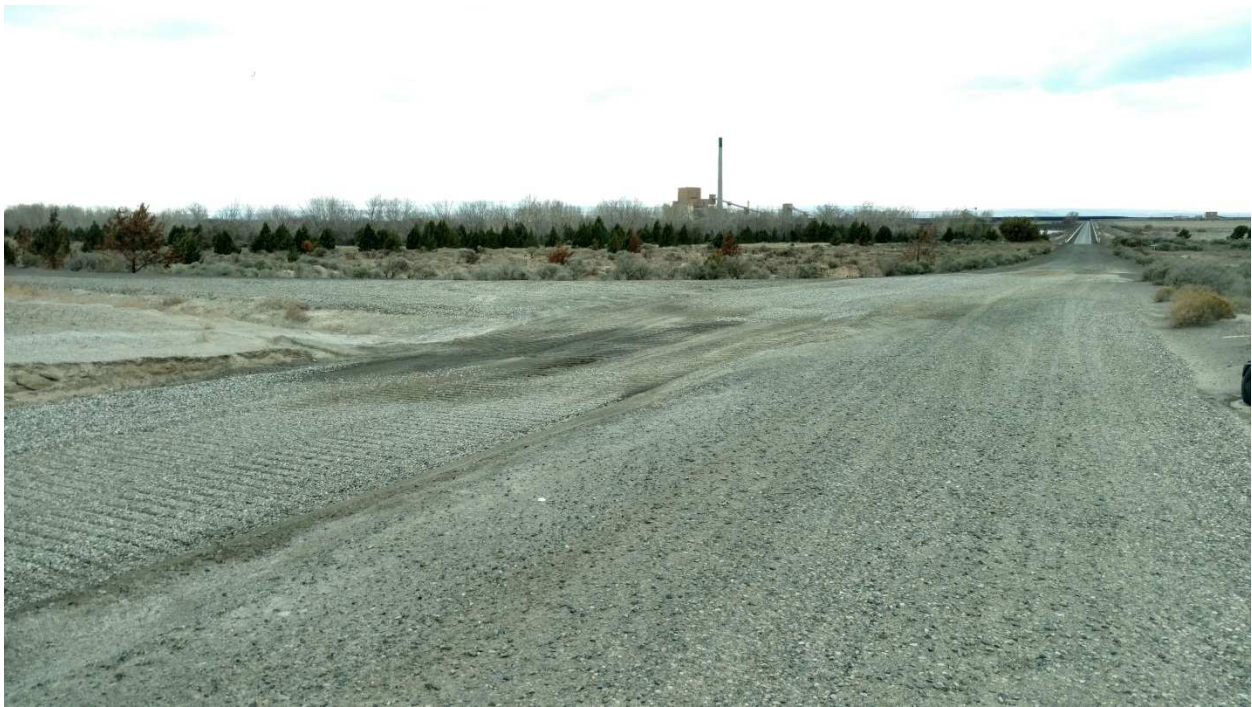
New gravel placed upon northeast vehicle entrance. Note: ditch profile to be maintained as new gravel materials compact with use.
